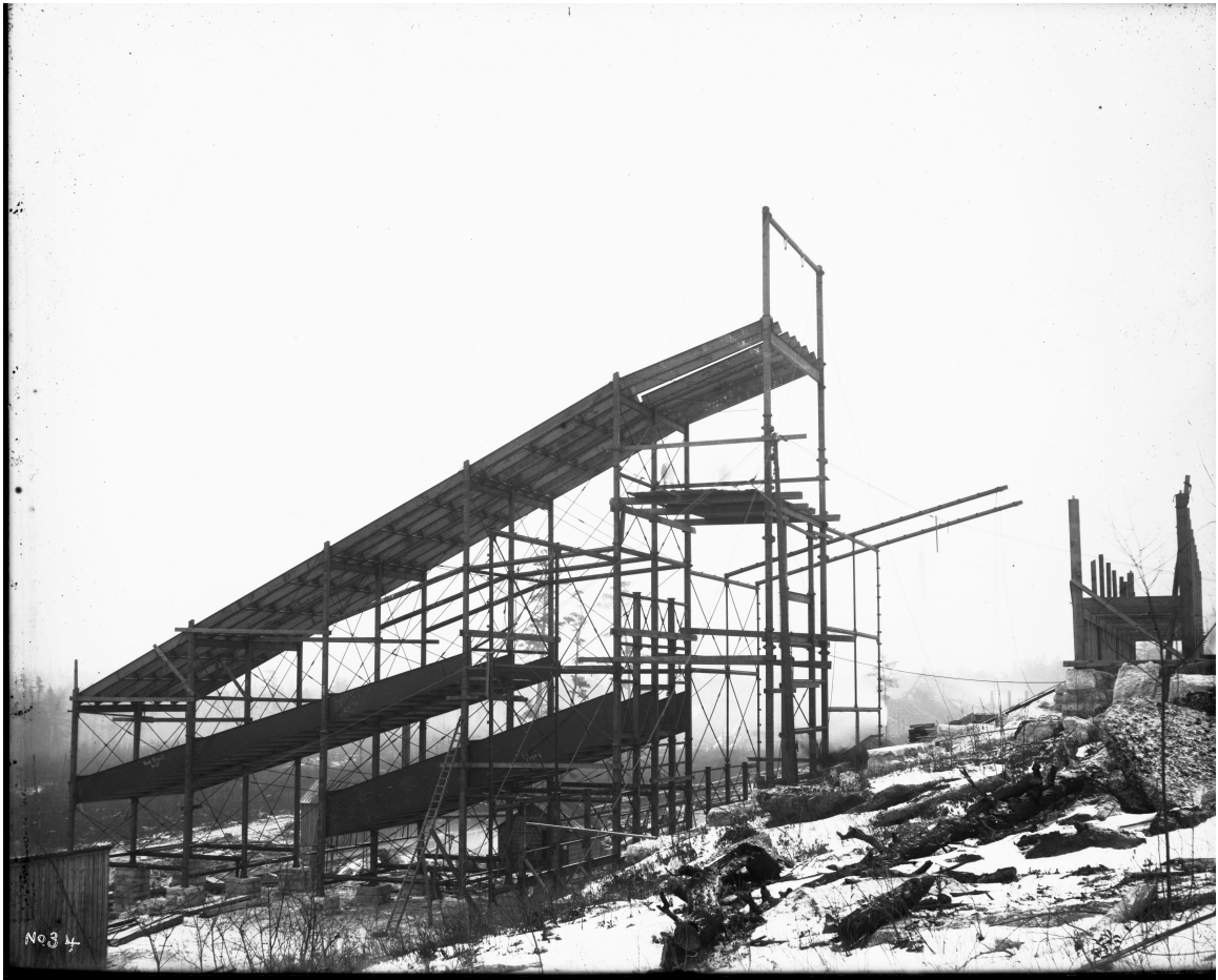
Figure 5.1: Iron breaker at Drifton, Pennsylvania, under construction about 1890. Negative 2-8, Coxe Collection, Division of Work and Industry, National Museum of American History, Smithsonian Institution. Scanned from glass plate negative by Eric Nystrom, 2006.
