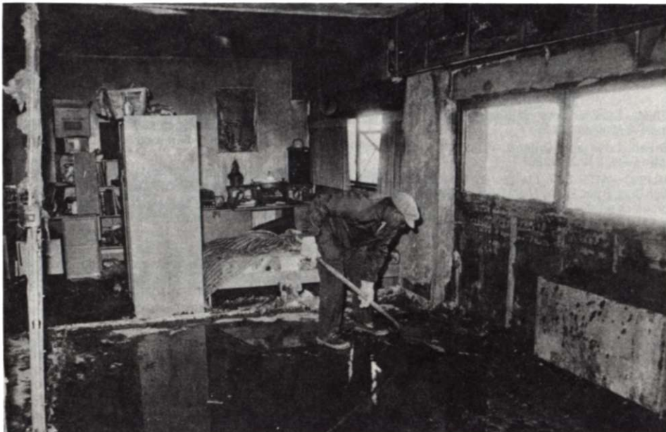
Cleaning up after the Tower A fire—what was once a suite.
