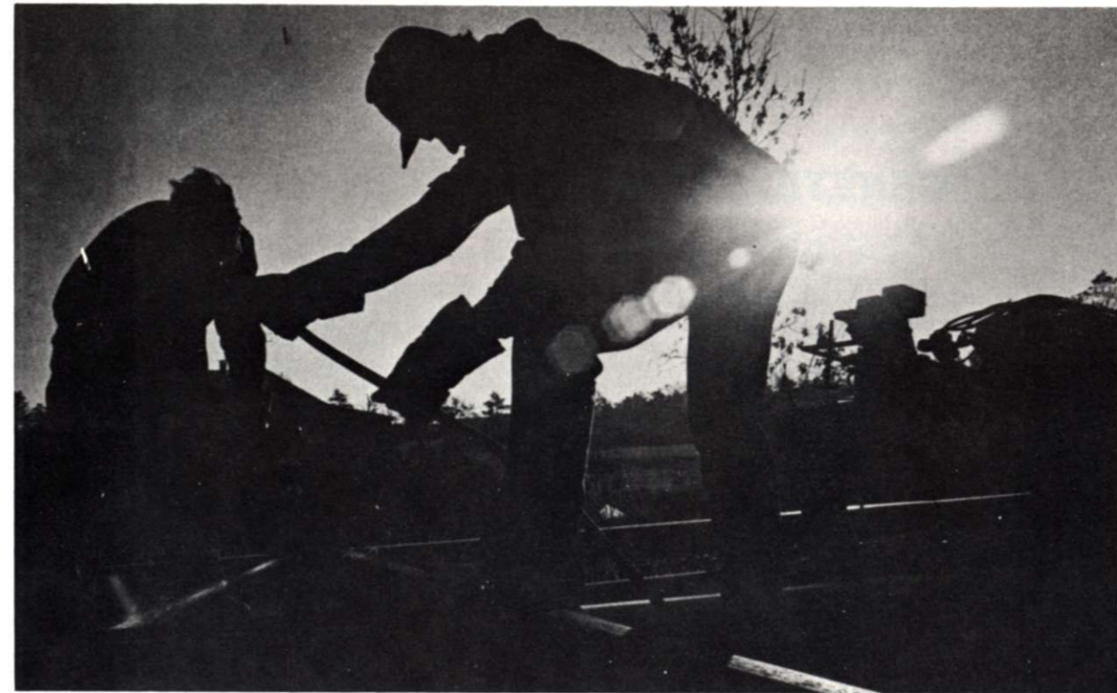
Two older track repairmen still enjoy working the rails and helping train the students.
