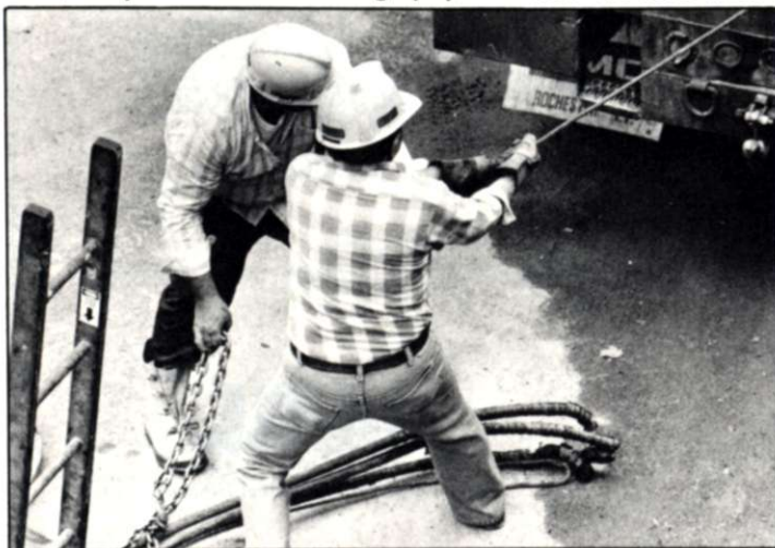
Workmen worked hard around the clock to bring power back to the campus.
