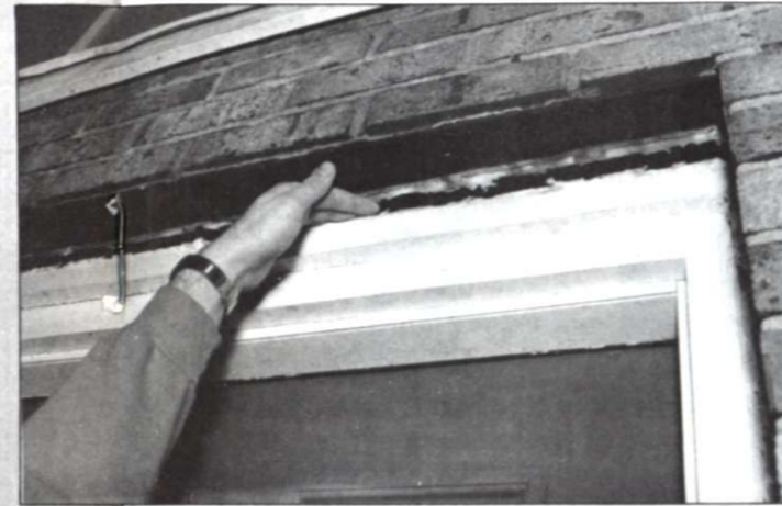
(far left) A would-be "thief" enters a townhouse through the closet crawlspace entrance. Placing heavy objects over it helps to remedy the problem.
