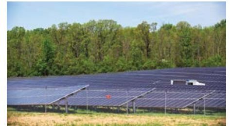
RIT's solar array can power the equivalent of 200 homes.
