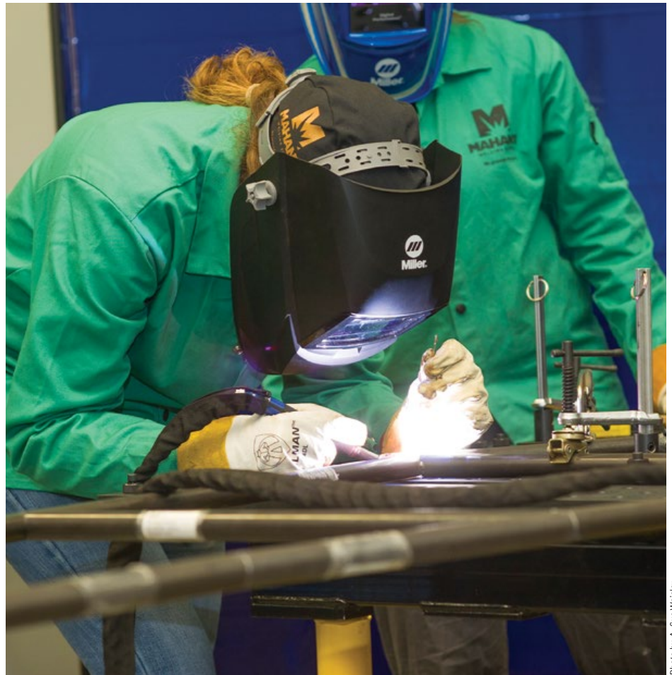
Zoe Bottcher, a second-year mechanical engineering major, welds the car’s frame at Mahany Welding. Six team members took welding classes at Mahany, which is owned by Michael Krupnicki ’99 (MBA).
