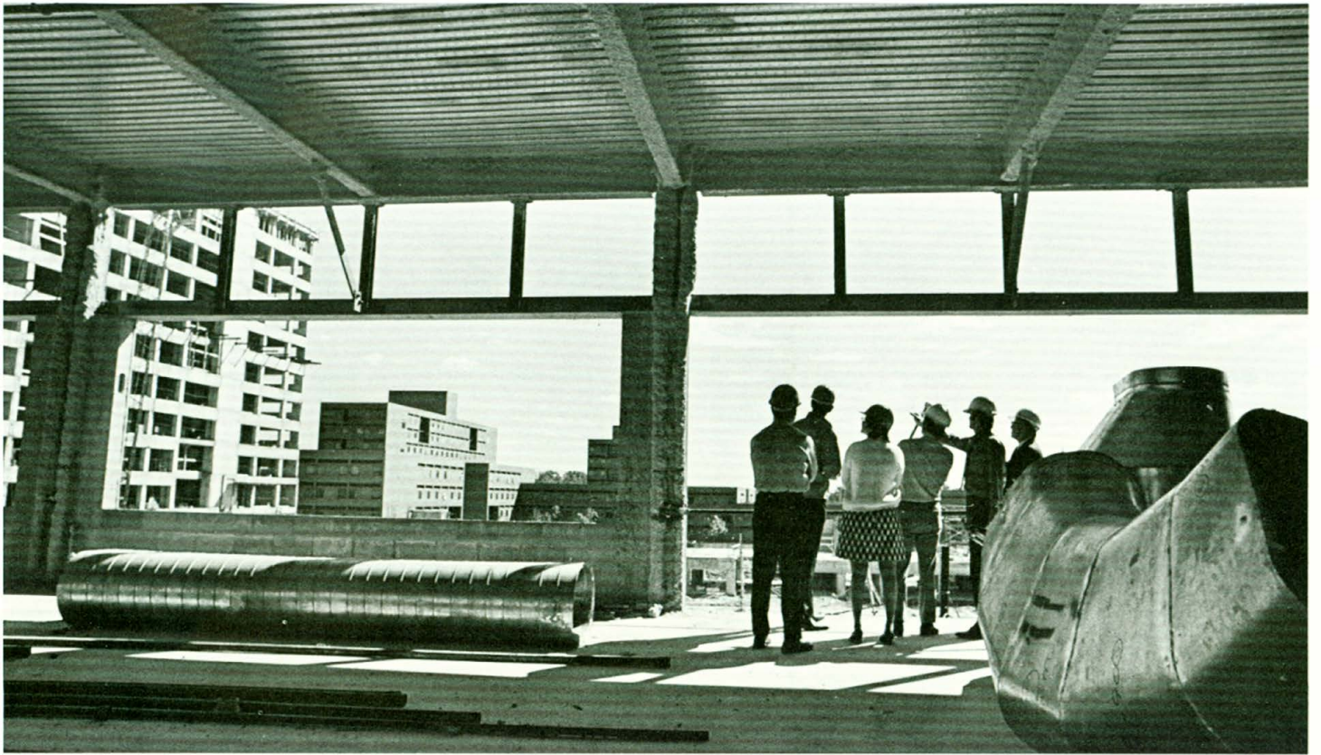
TOUR FACILITIES —Members of the NTID staff tour the facilities, looking over various phases of construction.
