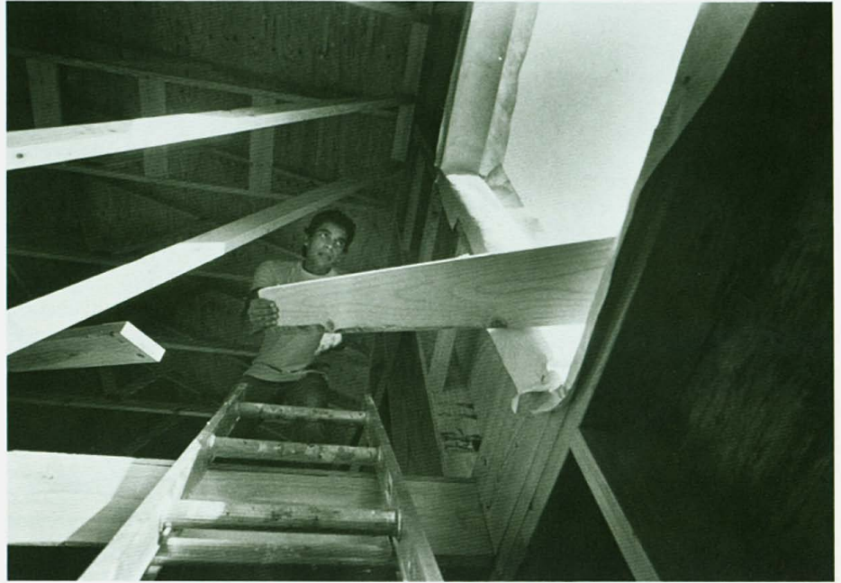
Putting on the finishing touches left and above, The Habitat for Humanity bouse on Hollister Street nears completion, thanks to the assistance of sorority and fraternity members.
