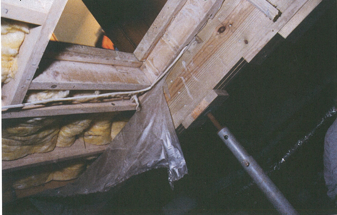
Racquet Club basement--don't use the jack holding up the floor to change the tire.
