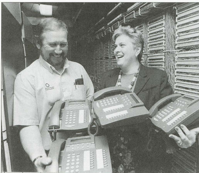
Lucent technician Gerry Costa, left, and Jamie Aymerich, operations manager for RIT Telecommunications Services, hold a few of the more than 2,000 new Lucent telephones installed on campus this summer.
