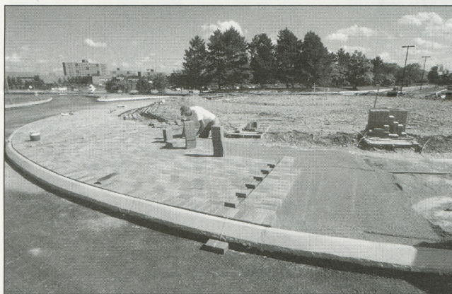
A worker lays brick pavers making up part of the new "roundabout" at Lomb Memorial and Andrews Memorial drives.
