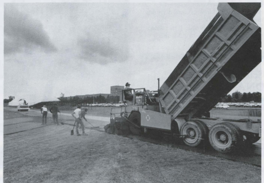
PAVING THE WAY...A work crew from DiFiore Construction Co. applies coating to RIT track. The quarter-mile track recently underwent a face lift and will be ready for general RIT use in mid-August.
