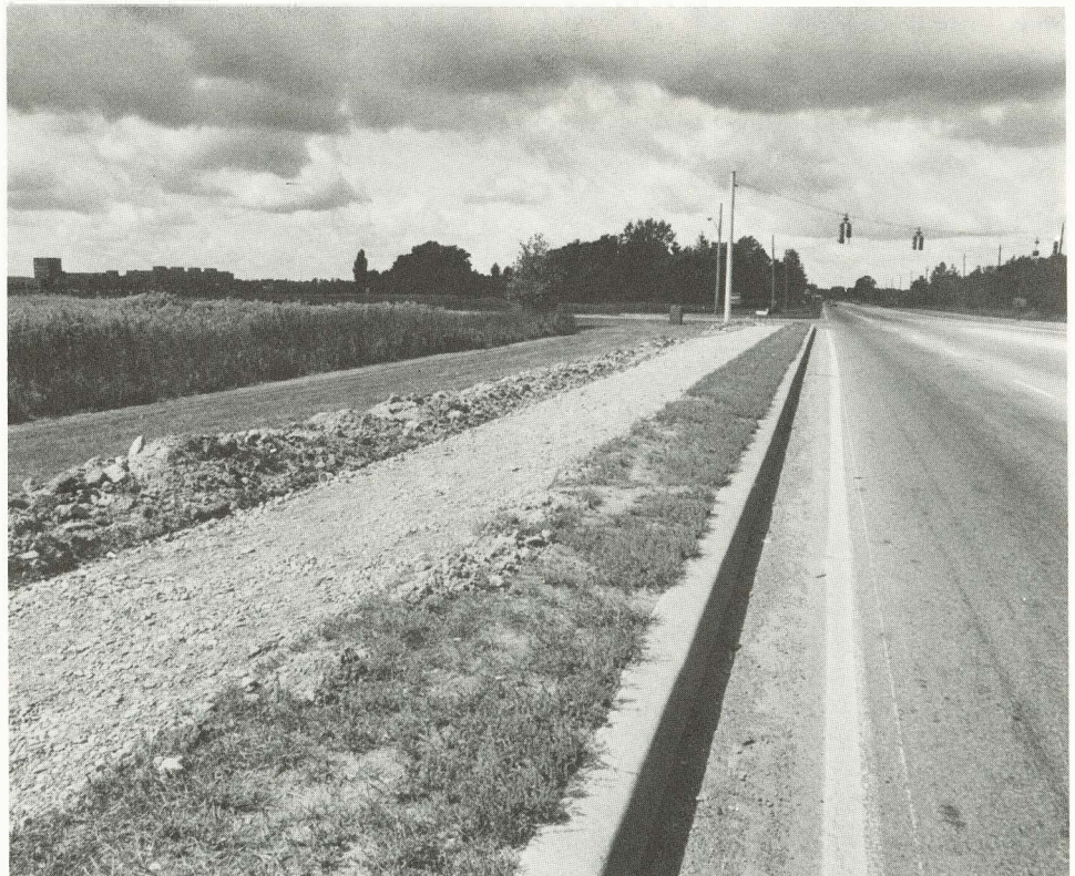
Almost done is the sidewalk along Jefferson Road running from Lowenthal Road on the eastern edge of campus to Southtown Plaza. The foundation for the sidewalk is ready for the top layer of asphalt. Target date for completion is October 1, according to the State Department of Transportation, which is having the sidewalk installed. The sidewalk is the result of requests to the State Dept. of Transportation from RIT's Office of Government Affairs and RIT students as well as the Town of Henrietta and State Assemblyman Jim Nagle. Next on the agenda for Jefferson Road is lighting, which is scheduled for 1981.
