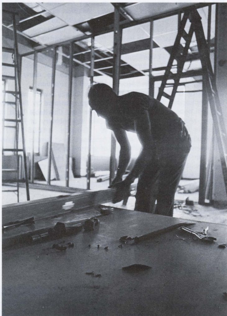
Workman building new offices on fifth floor of RIT administration building in preparation for large-scale shift of staff. See story, right.
