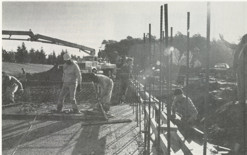
Let There be Concrete...Jim Scheetz, right, project manager for John B. Pike & Sons Inc., presides with majestic authority over the construction of the concrete pad that will serve as the foundation for the Kilian J. and Caroline S. Schmitt Interfaith Center. Pike & Son is construction manager for the project. The center, a 1,300,000-square-foot addition to the east side of the College Alumni Center, is scheduled to be completed next summer.
