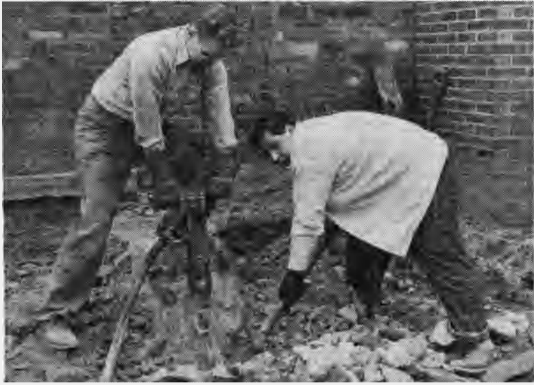
Excavation for the new Barracks Rec Hall was underway last week as workmen broke ground for the building's foundation. The cinder block structure will be erected against the north wall of the Crafts school. Pictured are Robert Hoff and Raymond Mazza, students. (Hayden Peake photo)
