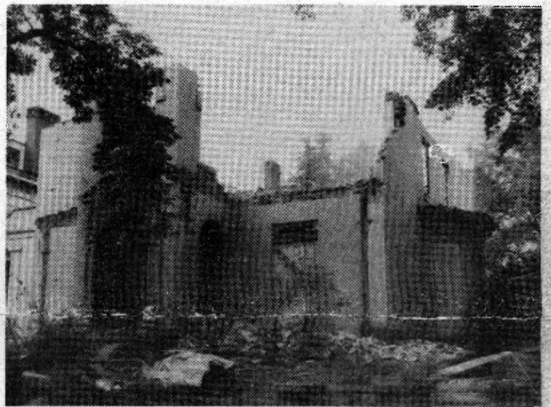
Progress toward the new gym has started in Livingston Park as one of the old houses is dismantled to make room for the new building. The Gym will be the first of five buildings to be built in the long range modernization and expansion plan under the 125th Anniversary program of the Institute.
