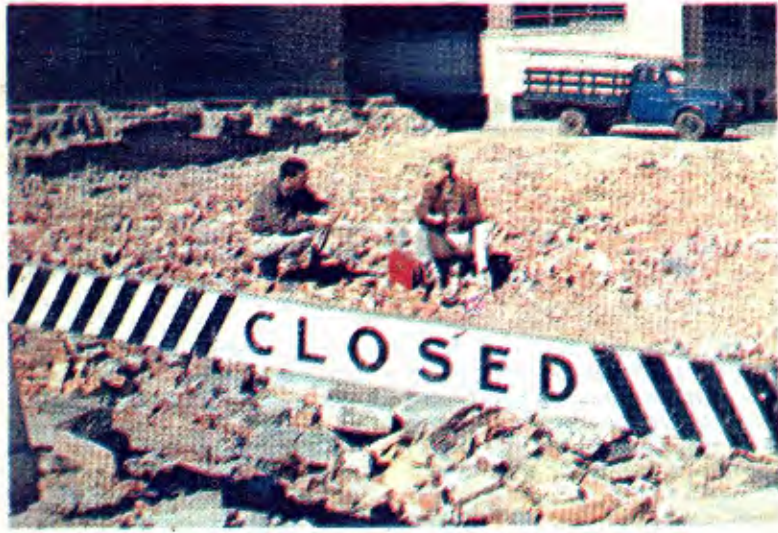
CLOSED IS RIGHT —And permanently, much to the pleasure of RIT's male population. This picture shows the site of the former men's dormitory at 102 Spring Street. All that is left are the bricks that were used to fill in the foundation of the old building. The demolition occurred over the past summer months. Benvenuto Bros., Inc., of Rochester, wrecking experts, handled the job. (Brown Photo)
