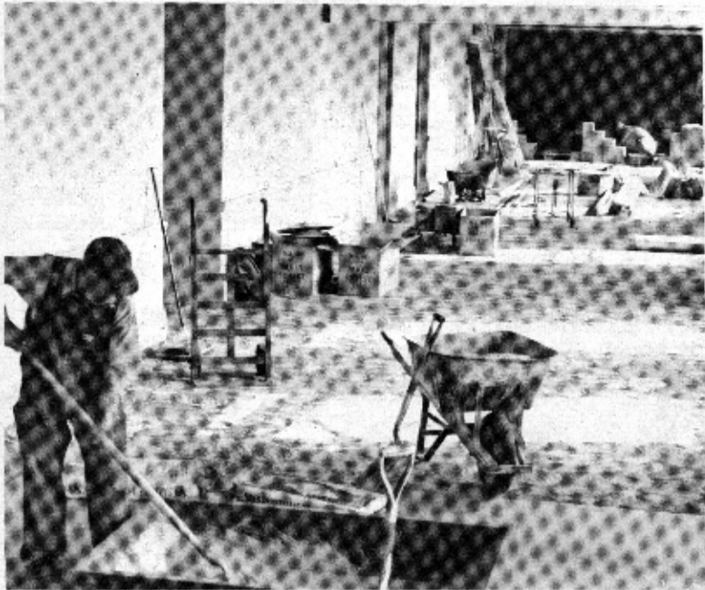
ROOMS FOR RENT—Workman begin renovation of the third floor meeting rooms in the Men's Dorm. Upon completion of work the dorm will house all male freshman and sophmores
