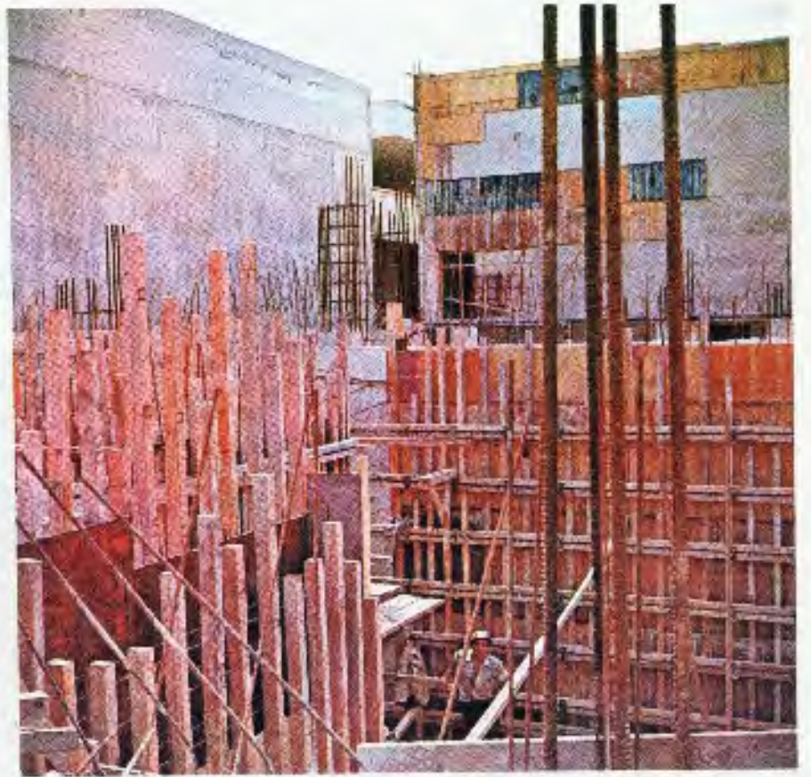
Supports are still being used in the lower levels of the College Union as progress on that building creeps along.
