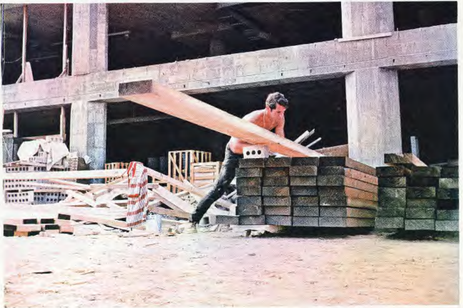
A workman cuts a support beam for concrete molds used in the Graphic and Applied Arts Building.
