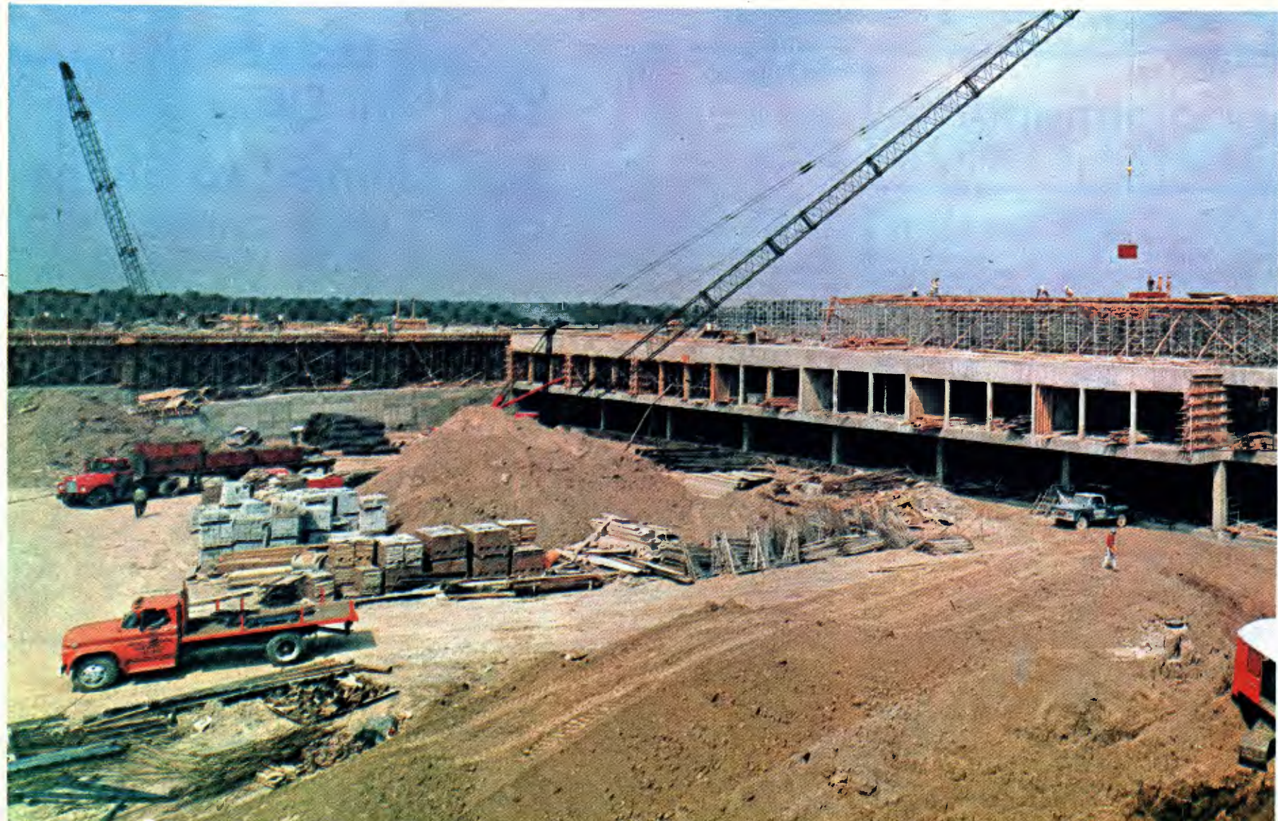
GROWTH —The rapid progress made at the new campus during the summer months is readily apparent in this photo of the Fine and Applied Arts, Graphic Arts and Photography building complex. This view is from the Business, Health, and Administration building over one of the court yards that will enhance the campus.
