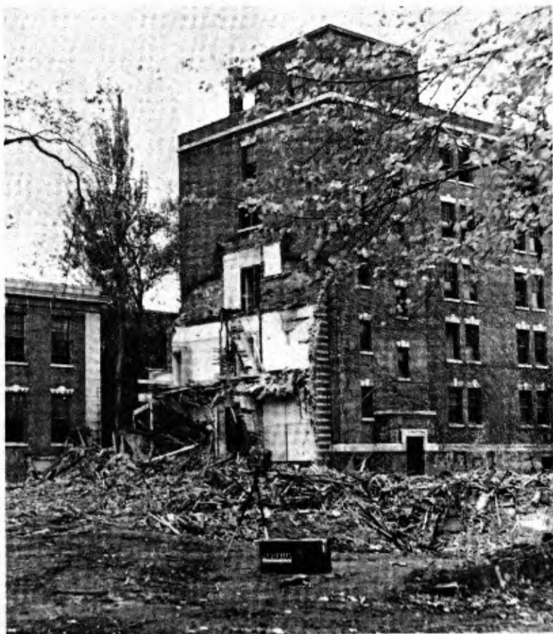
ONLY MEMORIES REMAIN — Perkins Hall, an RIT women's dormitory for the past two years, is no more. Wrecking crews have been at work for the past several weeks tearing down the old buildings to make way for an urban renewal project. This view is looking in from Main Street across the front lawn. (Photo by Harry Schaefer)
