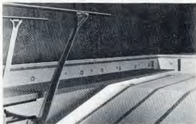
COLLEGE UNION POOL—Finishing touches are being made on the olympic-size swimming pool at the new campus. (Staff photo by Nick Morgan.)
