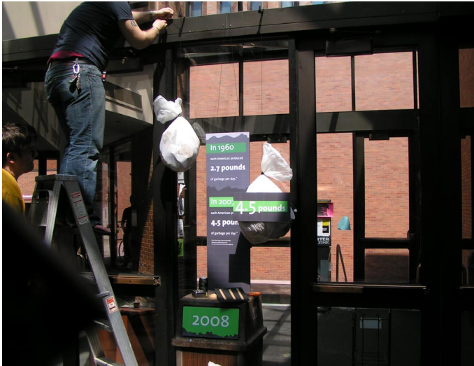
Solution Three installation
