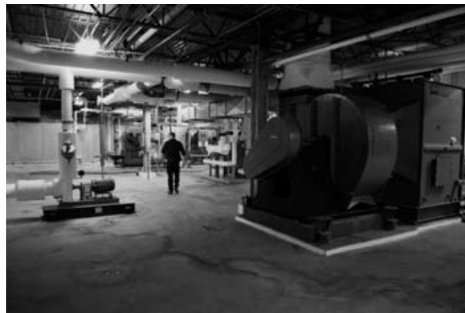
Below: Ed Davin, HVAC/R Technician makes daily rounds to all boiler and chiller rooms on campus, making sure everything is running properly.
